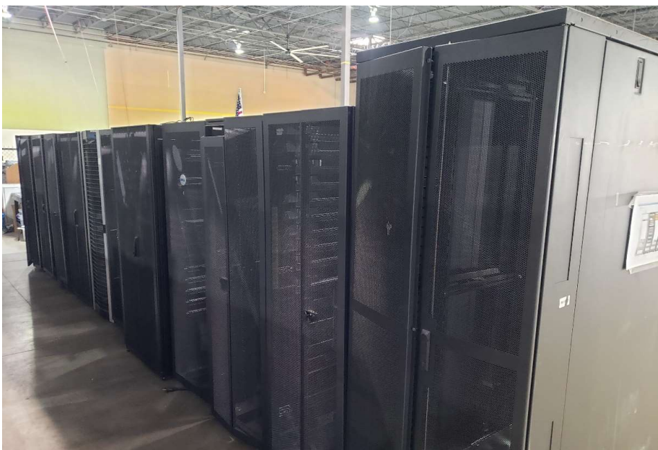
42U and 48U Server Racks
